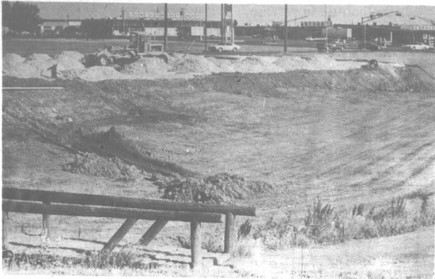
A site in the 1200 block of N. Hobart is being readied for the construction of a 7-Eleven convenience store and a Long John Silver's sea food restaurant. The two buildings will be side by side. Construction costs on the
