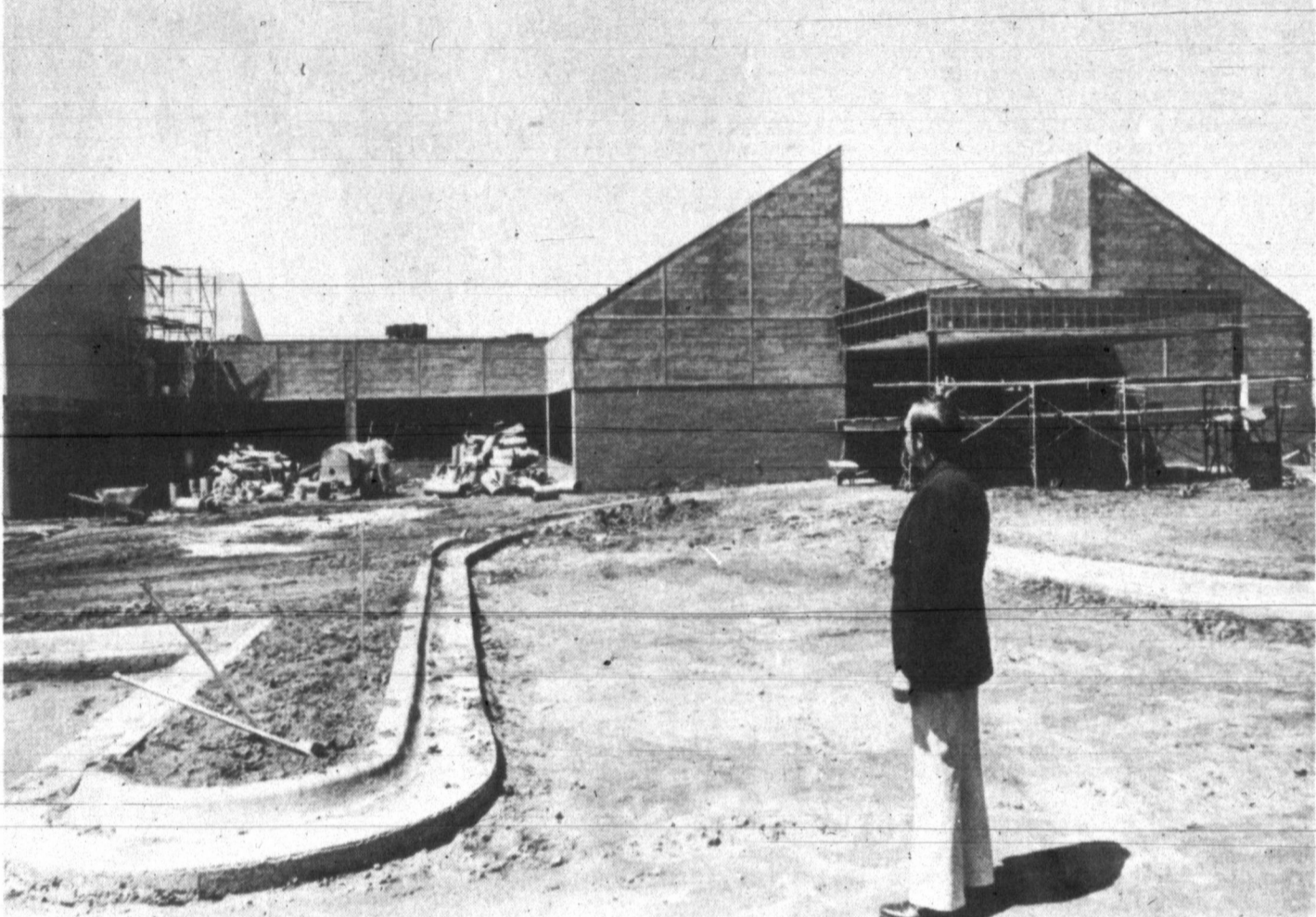
NEW COUNTY HOSPITAL — Tony Weatherly, hospital administrator, looks at the $1.5 million Hemphill County Hospital well under way in Canadian. The 27-bed hospital is designed so that it can easily be expanded to 50 beds.
