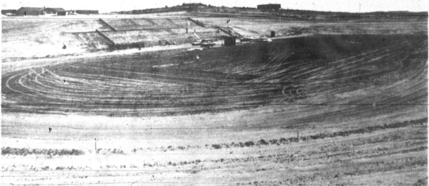
NEW BOWL — Canadian's new football stadium will seat 2,000 home fans and 1,000 visitors with room on the slopes for many more. The stadium is part of a $3 million plus addition to school facilities. Canadian is clearing ground for a new high school. Joe R. Cullender, superintendent of
