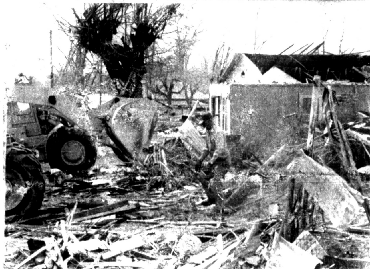
CLEANING UP — A few short hours after a third of the town was reduced to rubble, Lefors people and hundreds of volunteers began cleaning up and repairing. (Pampa News Photos by Thom Marshall)
