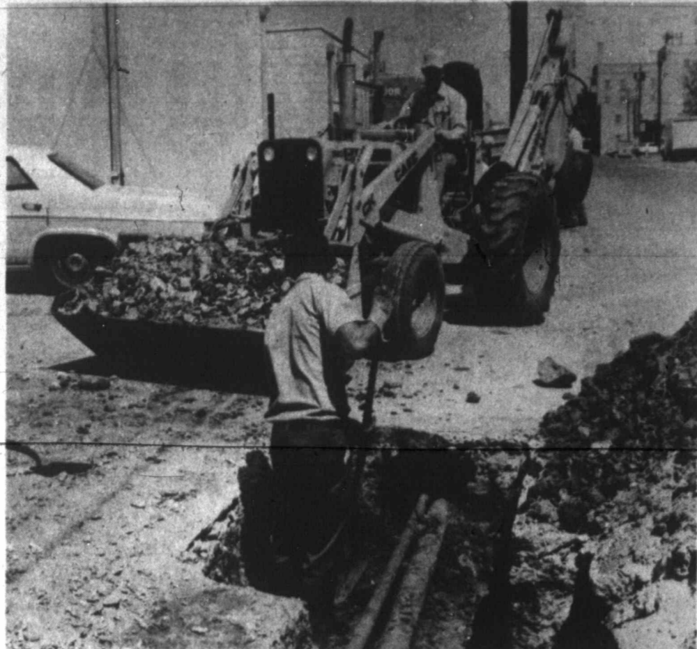
SAFETY CHECKS are a continuing program with Pioneer Natural Gas Co. Ricky Davis operates a front loader as Gary Montgomery cleans out the excavation. The location is on West Foster where a two-inch and a four-inch lone are inspected for leakage. (Photo by Frank Bain)
