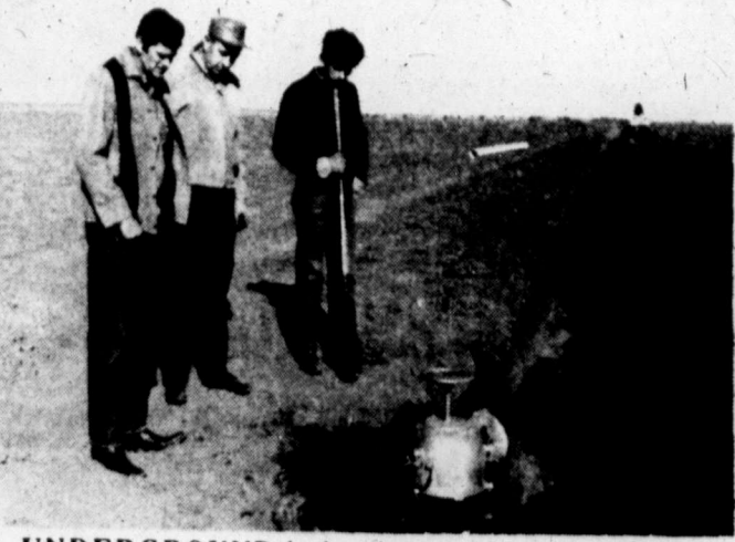
UNDERGROUND irrigation pipeline on a Gray County farm northwest of Pampa is inspected here by Jim Roach, left, Foster Whaley, and an unidentified worker. The underground installation has many advantages, including conservation of water.
