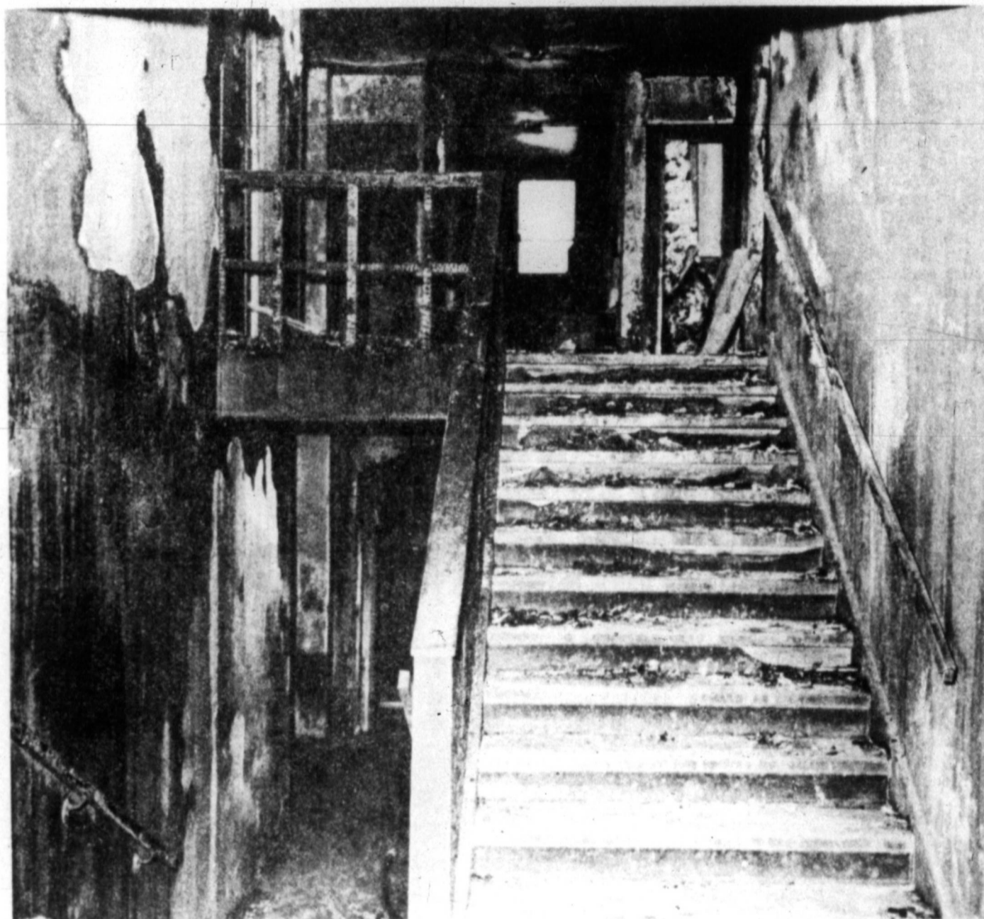
BLACKENED STAIRS lead up to the offices behind the sanctuary
