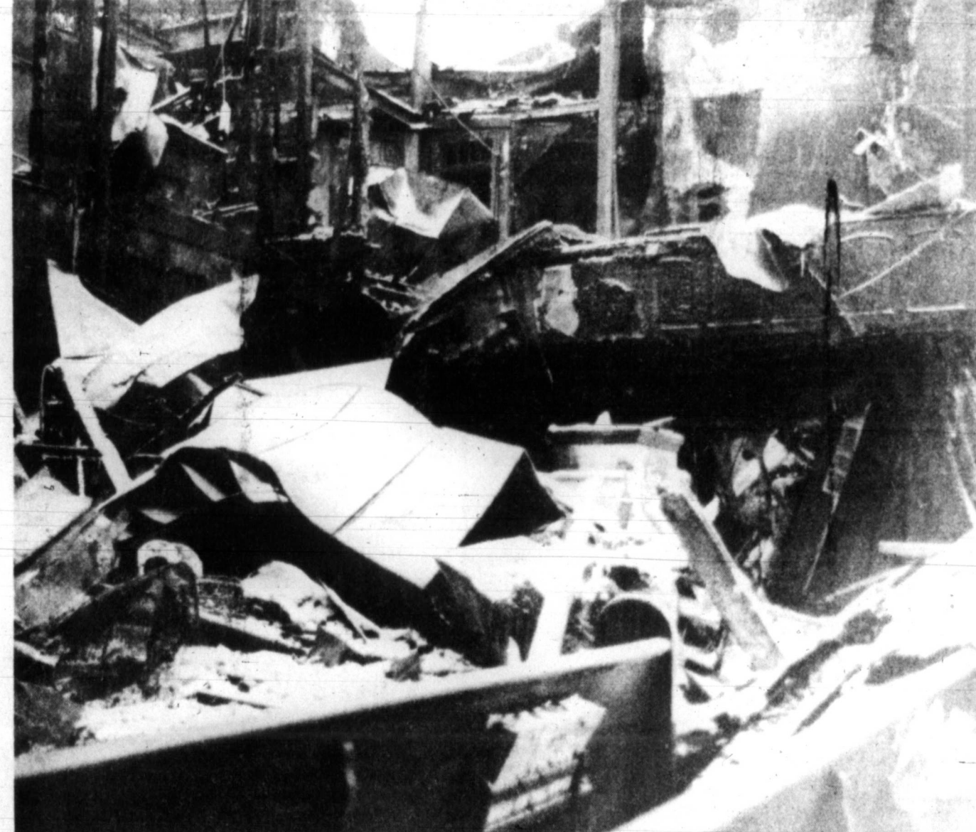
IN THE AFTERMATH — Snow covers the remains of the sanctuary at First Baptist Church after fire razed the structure Sunday night, with damages possibly exceeding $1 million. Officials are still working to determine the cause of the blaze. (Photo by Terry Hanna)
