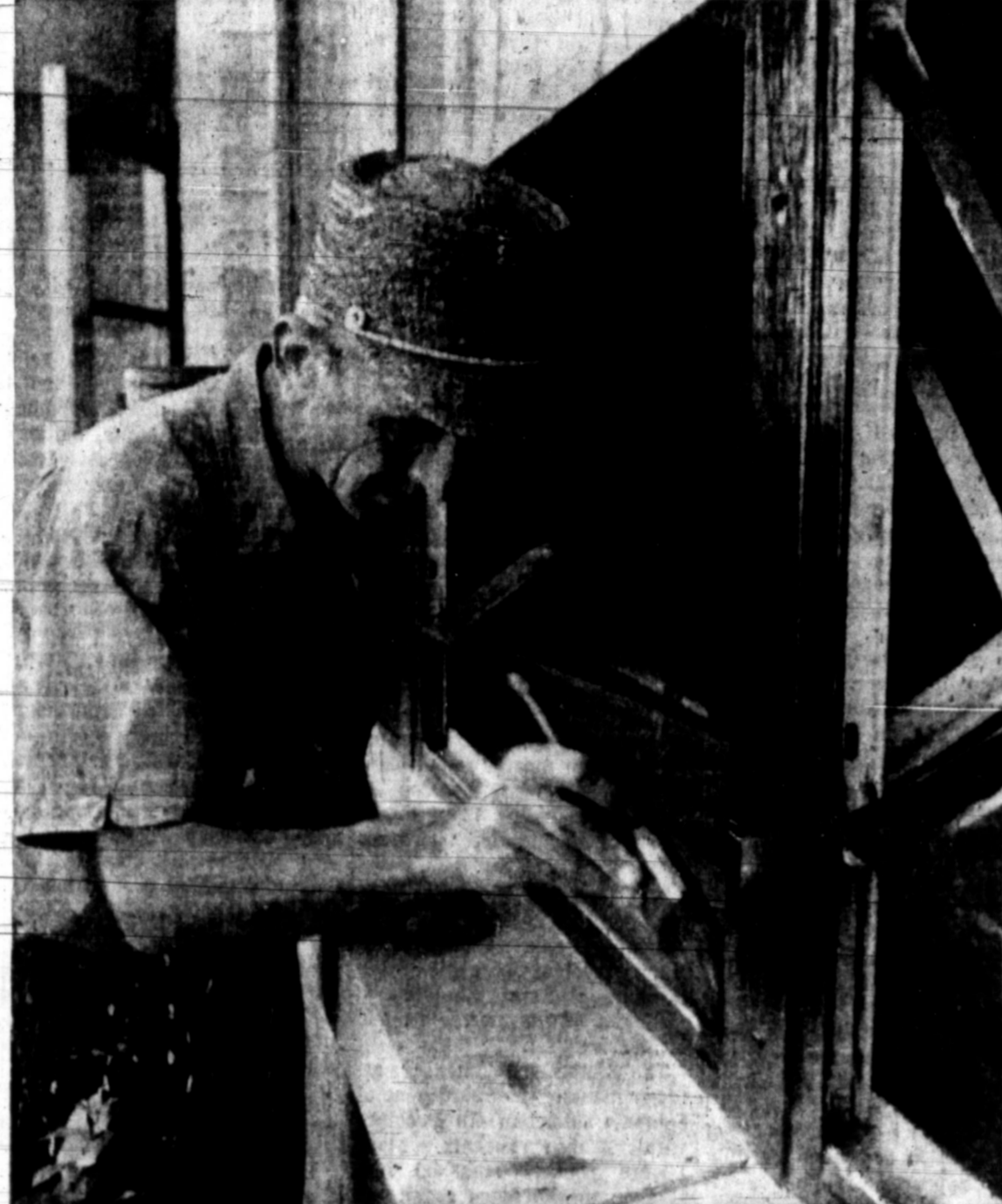
ACTIVITY AROUND Pampa schools is getting in high gear as buildings and classrooms are readied for the influx of more than 5,800 students expected on the first full day of school, Tuesday, Sept. 2. Pictured adding a fresh, new look to Stephen F. Austin Elementary School is a "Rembrandt With A Paint-Brush," Wendell Watson, Pampa High School biology instructor. (Staff Photo)
