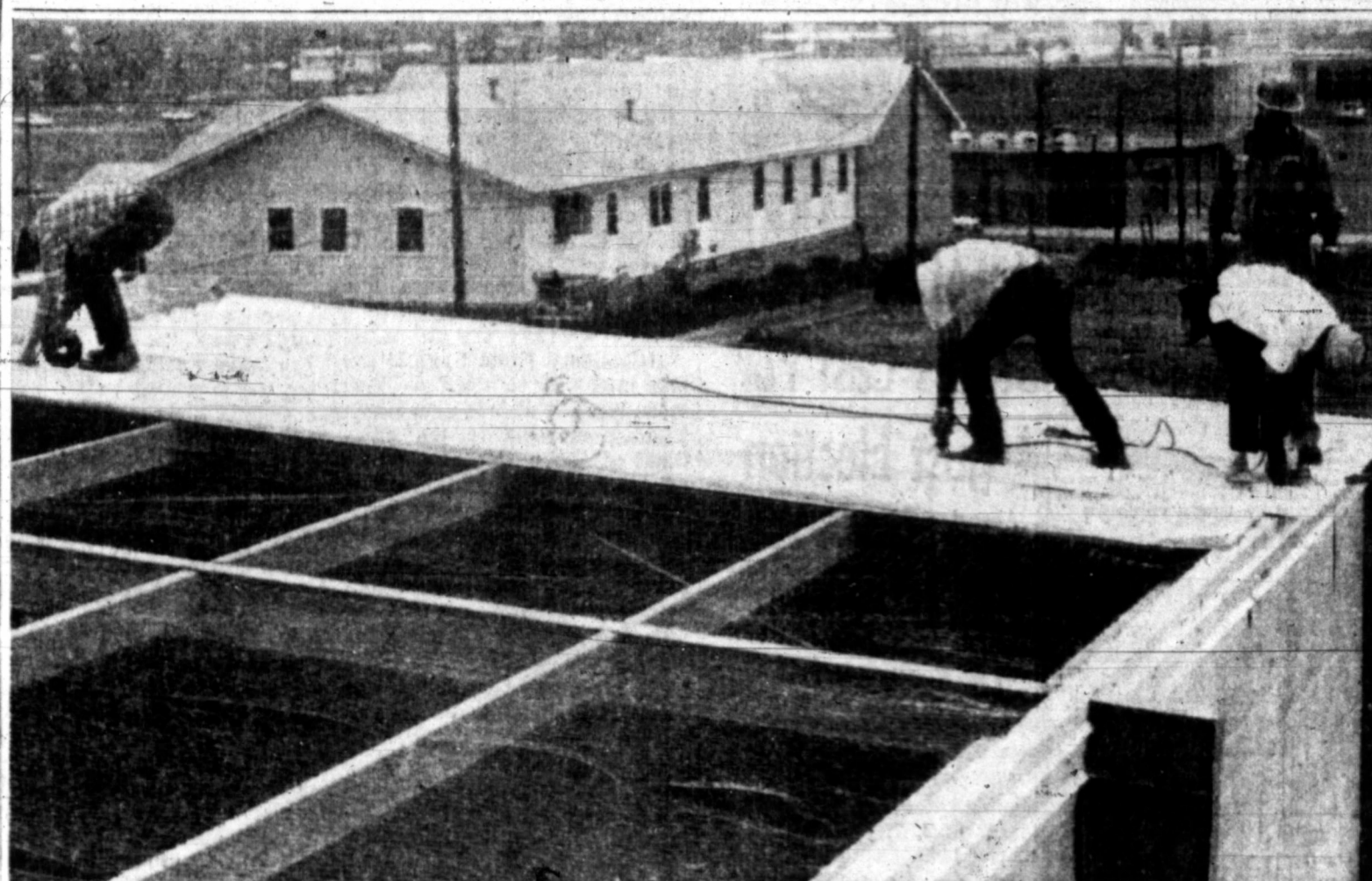
ROOF FOR HEALTH CLUB ADDITION —Workmen for Pam-Tex are putting the finishing touches on the roof for the new health club addition to the Pampa Youth and Community Center. The new addition, which is located on the east side of the present building, will include a modern, well-equipped health club and two regulation handball courts.
