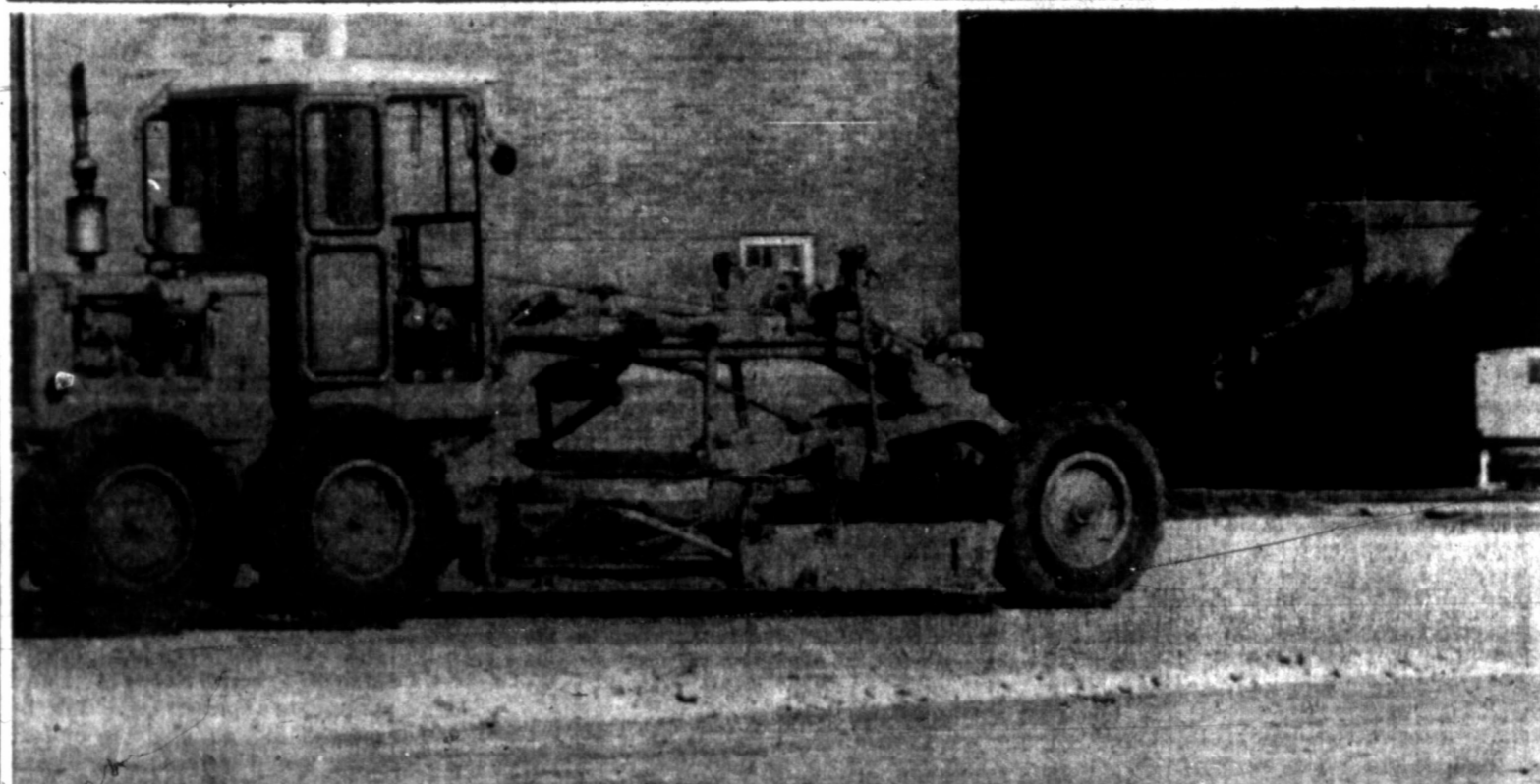
PAVING WORK GETS UNDERWAY — Workmen are busy filling in the playground area at Pampa Junior High as the first step toward paving the corner lot. Downtown merchants are paying part of the cost of the
