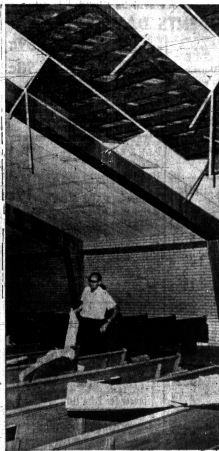
SAFETY IN TIME OF STORM — Churches are supposed to be a place of safety in time of storm but anything can happen at other times. Such was the case Wednesday night when part of the suspended ceiling at the Fellowship Baptist Church fell into the back part of the church. Luckily, evening services had been dismissed earlier. Rev. Earl Maddux was busy Thursday morning trying to get the church cleaned. (Photo By Bob Kelly)
