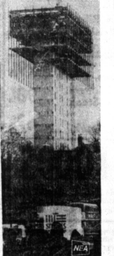
COMING DOWN? No, it's going up, but scaffolding on this new building in London makes it look as though it were being demolished instead of being constructed from the ground up.
