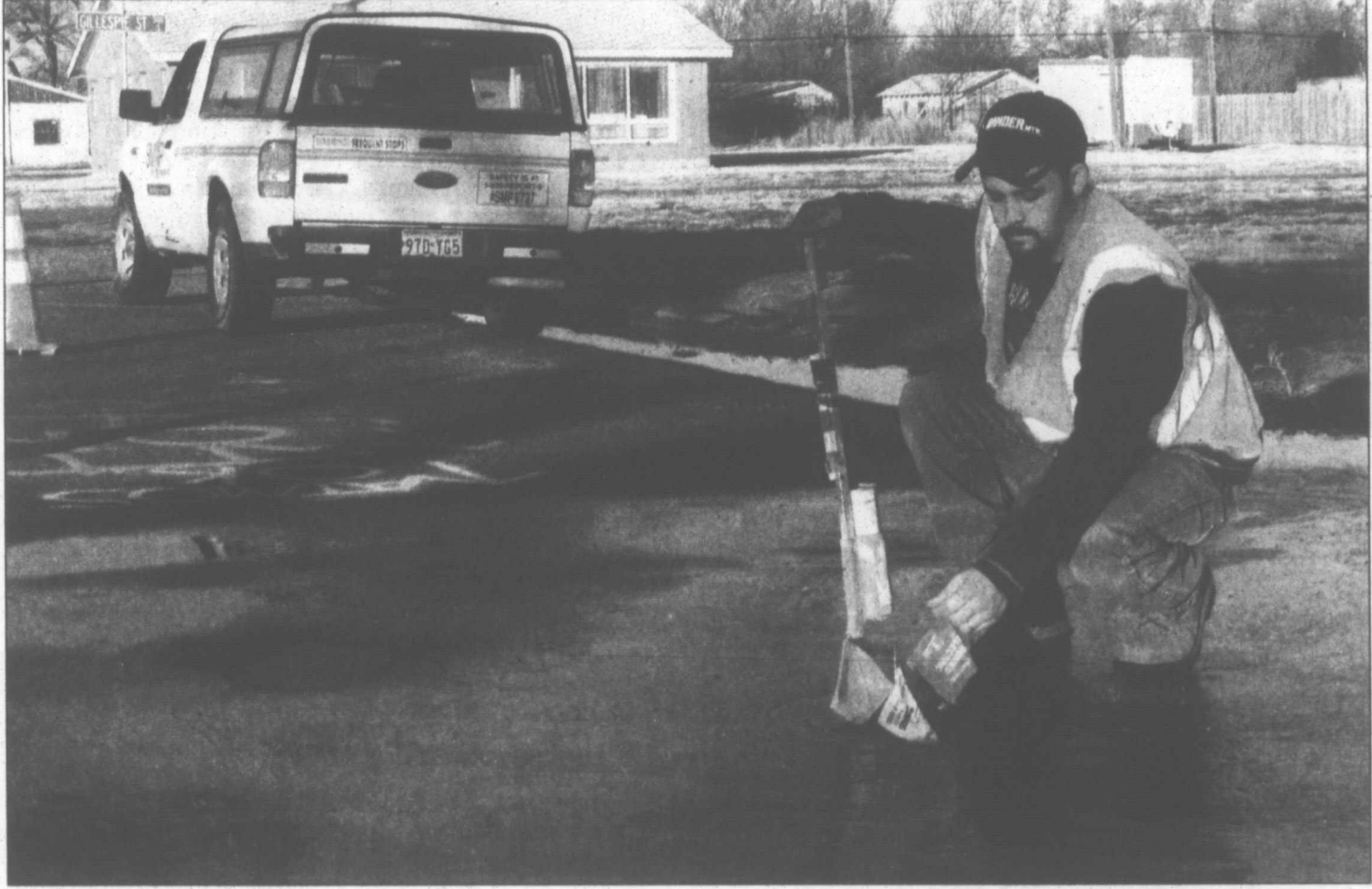
Pampa News Photo by KERRI SMITH Ryan Milligan from SM&P places flags and paints the roadway to show city workers where utility lines are located underground before they start digging to fix a water main break.
