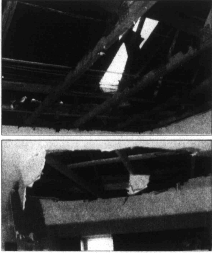
Pampa News Photos by JORDAN REAGAN Top photo - A hole remains in the roof of an apartment after Tuesday's fire at the Courtyard Apartments. Bottom photo - The adjacent apartment sustained damages to the ceiling.
