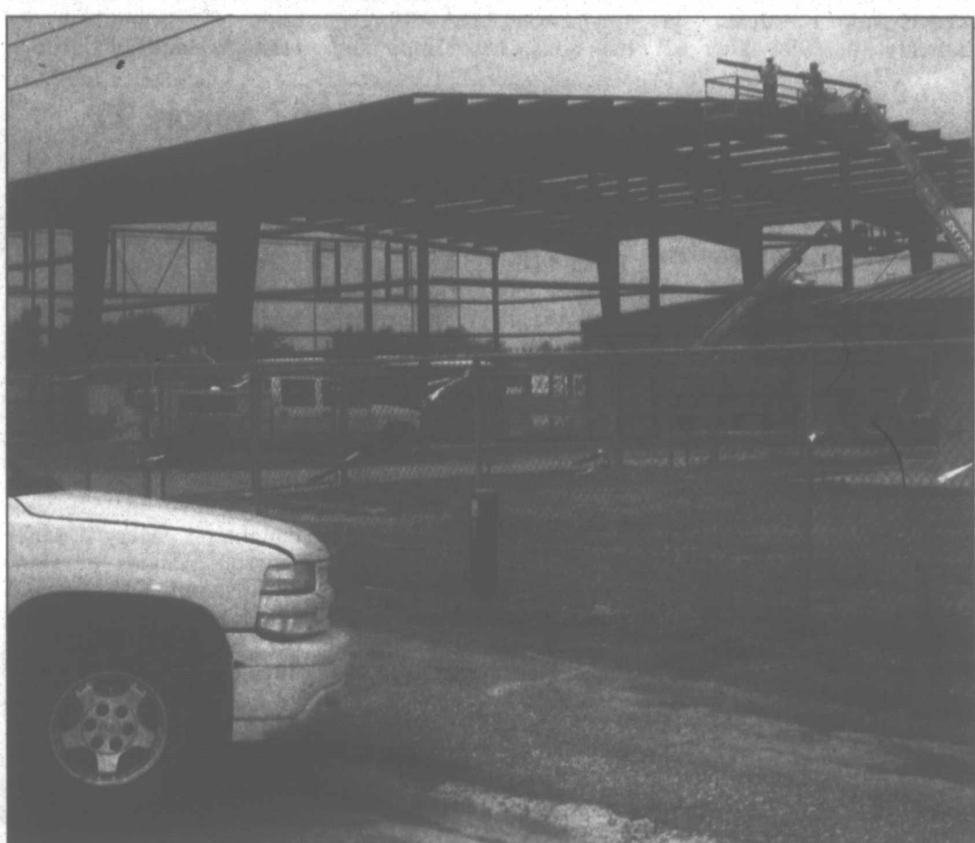
Steel is being erected on a new concrete slab in front of the MPAC building at Pampa High School, part of the renovation and construction at the high school thanks to the bond election that passed last year.
