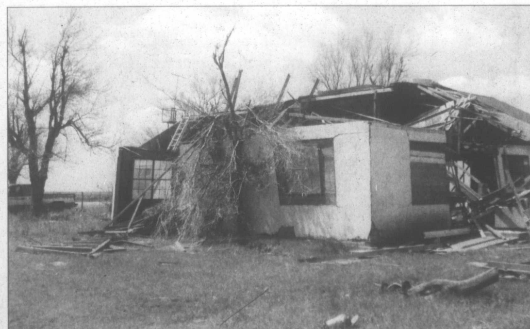
The back corner of the Wills home is still standing as are several trees nearby.
