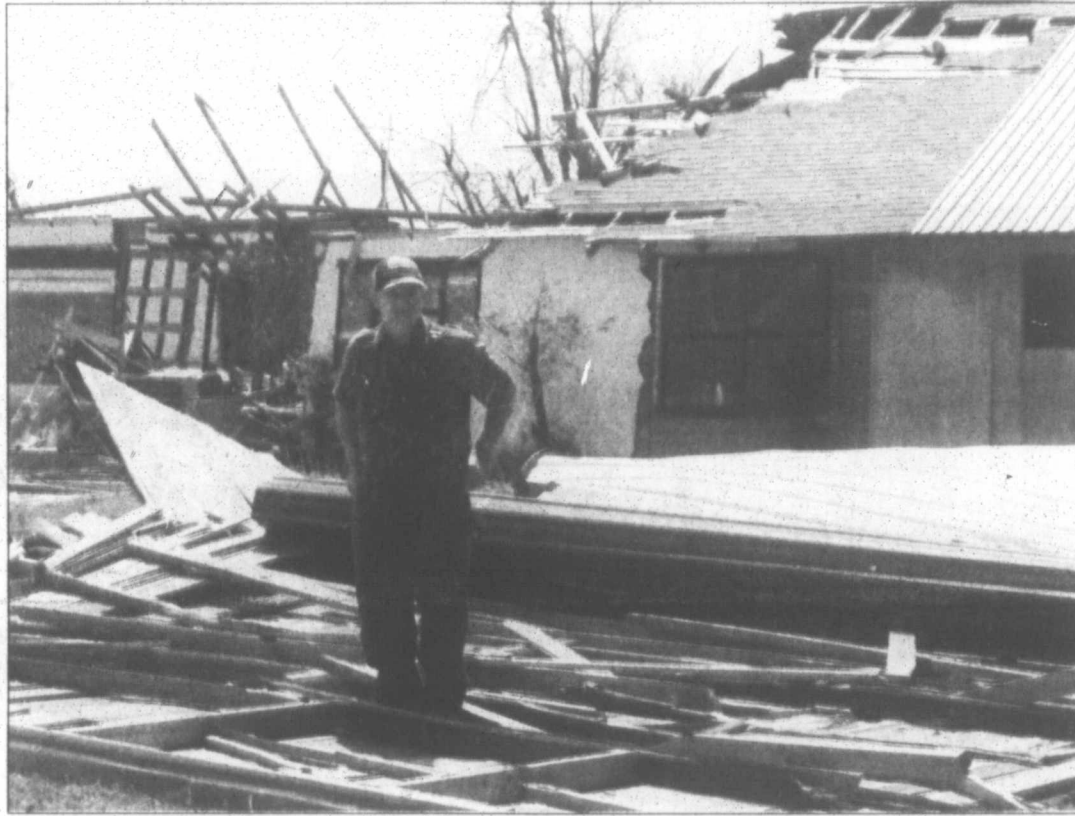
Melvin Wills stands on what used to be the roof of his house after a tornado struck April 21.
