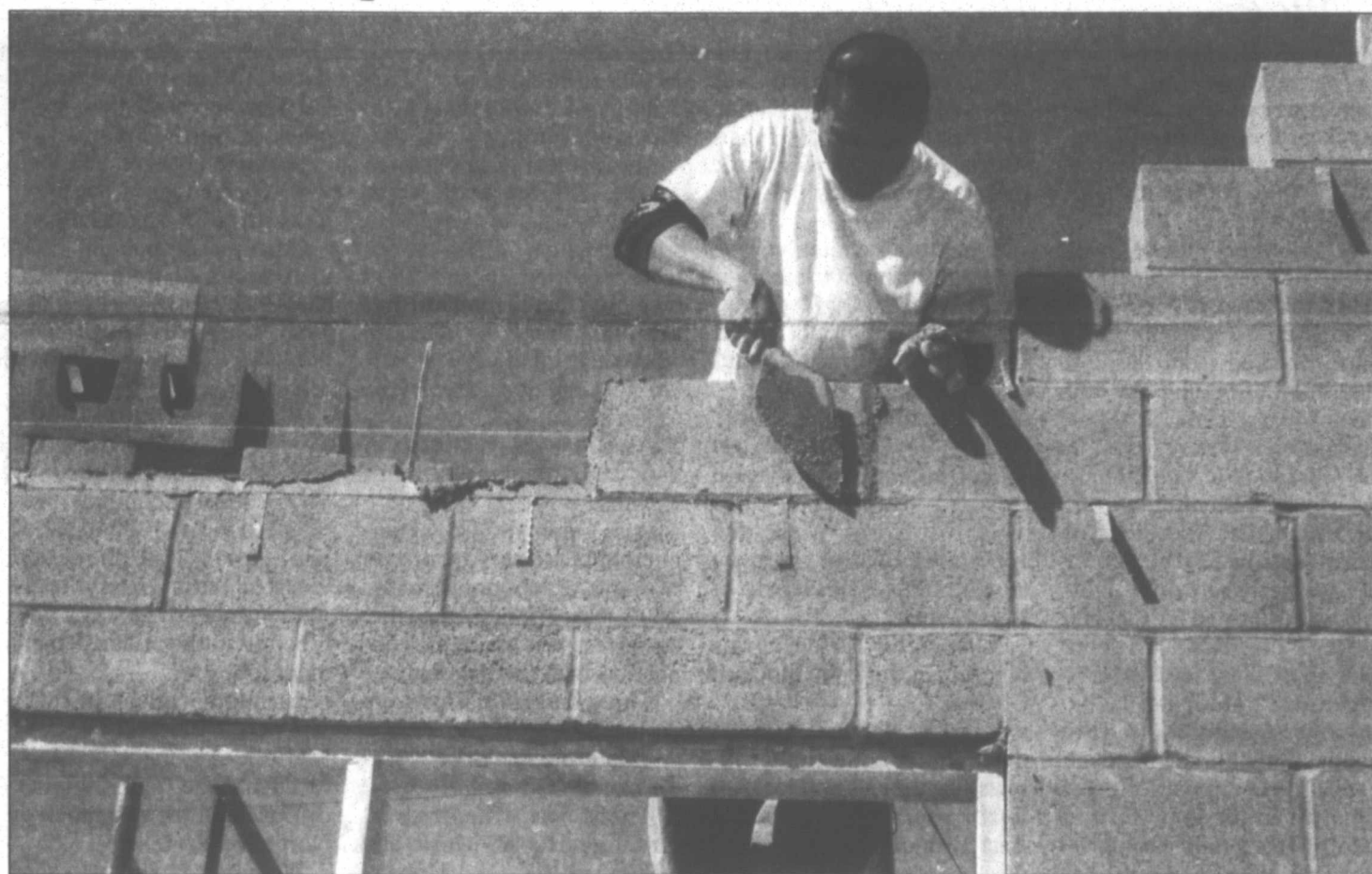
Pampa News Photo by KERRI SMITH Witt Masonry from Amarillo is the company setting the blocks and bricks on the new office building for Quality Sales on North Hobart. T.J. Cobos is shown smoothing out the mortar between blocks.
