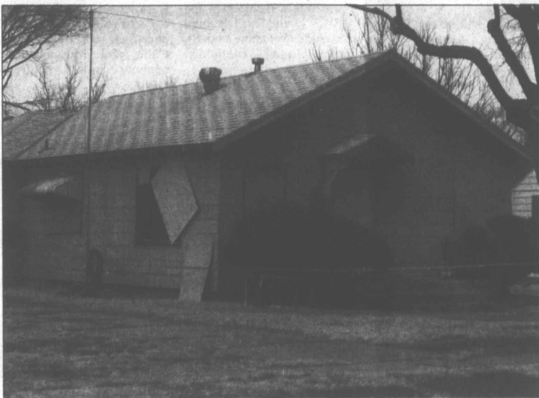
Pampa News photo by MARILYN POWERS A leak in ductwork from a floor furnace over the years caused a decomposition of material around a floor joist that started a fire at this home at 1029 Twiford Saturday morning. Chong Janeway, 47, died in the blaze.
