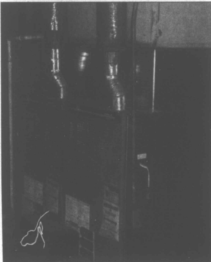
Pampa News Photo by KERRI SMITH Gas heaters like this one should be cleaned and checked regularly. To avoid carbon monoxide poisoning, it is important to make sure fumes are vented properly through ventilation pipes leading outside.
