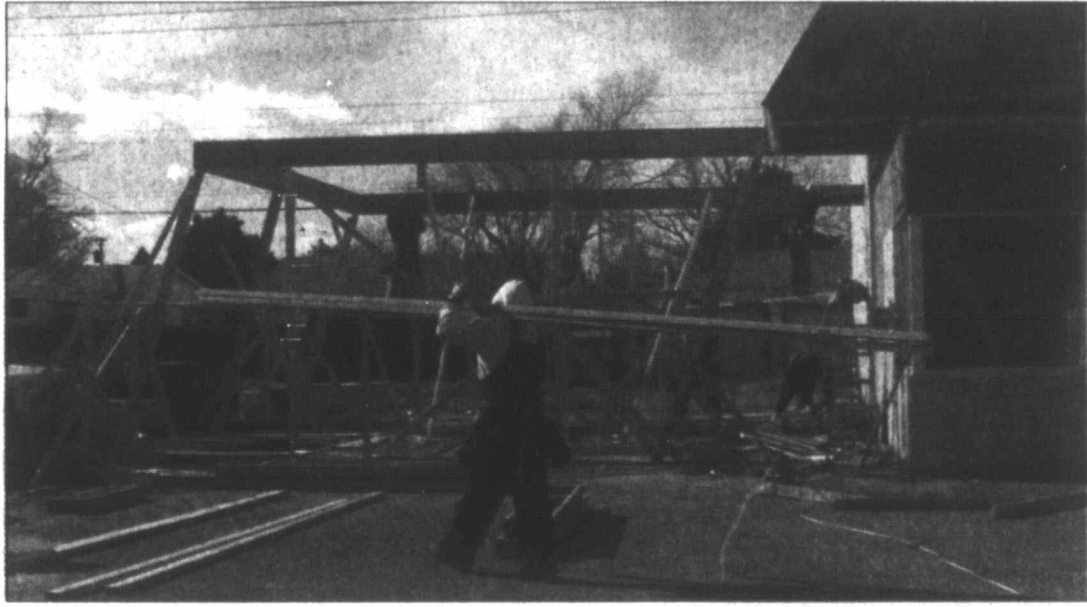
Pampa News Photo by KERRI SMITH A crew from Fuller Framing from Amarillo added on to the old Royse Animal Hospital at 1939 N. Hobart last week. Once construction is complete in about one month, the building will be the new home of a branch of Pamcel Federal Credit Union, according to the general contractor on the job, Bob Sanders from Sanders Construction.
