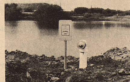
The first dry hydrant in West Texas was installed at Gail by Upper Colorado SWCD and Big Country RC&D. The dry hydrant gives rural fire departments quick and easy access to a water supply. Several more of these hydrants are planned for Scurry and Borden counties.
