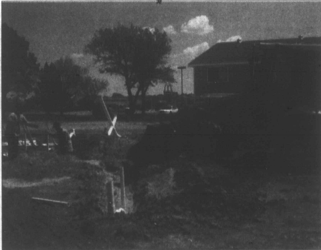
Pampa News photo by REDONN WOODS Matt Parks, left, and Scott Hudson work the trenches while Johnny Williams mans the backhoe for Larry Baker Plumbing, Heating and Air. The crew was working on a conference center that will complement Americinn and overflow from M.K. Brown auditorium, according to contractor Chuck Morgan.
