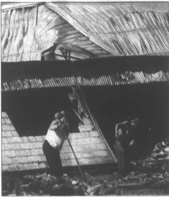
Pampa News photo by MARILYN POWERS Regina Ellis, left, and Alejandro Estrada begin cleanup operations this morning at the site of W & W Fiberglass Tank Company's burned building at 207 S. Price Road.
