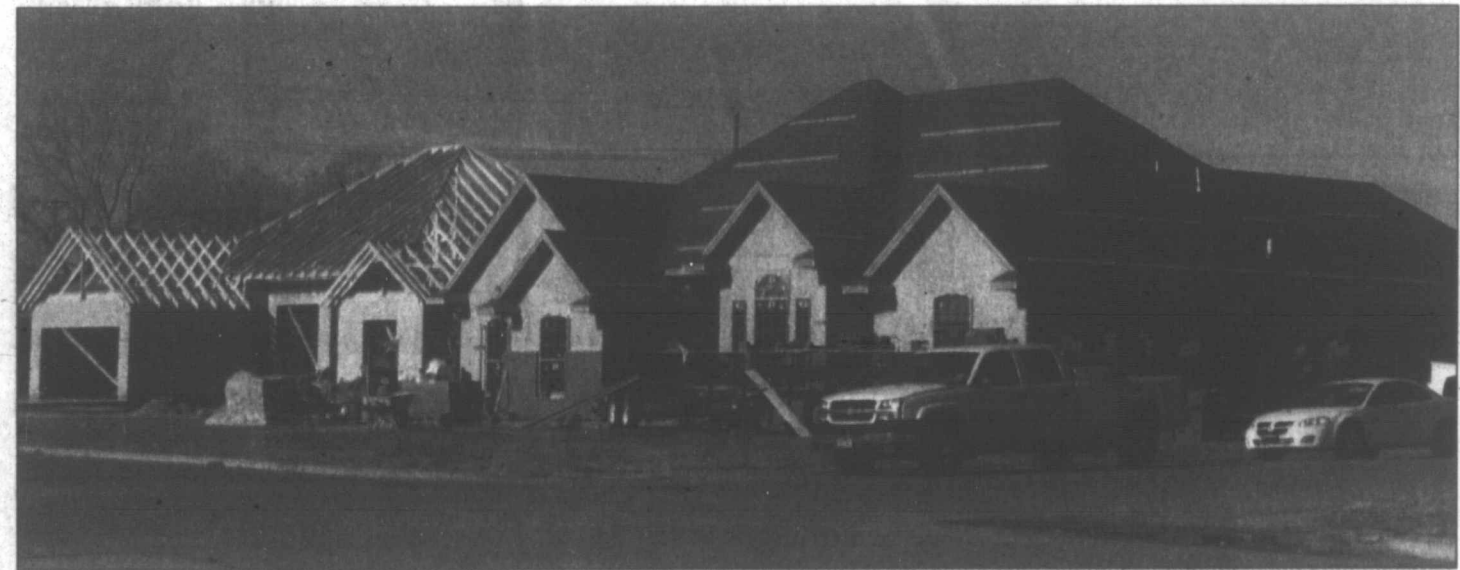
Pampa News photo by MARILYN POWERS Work progresses on two houses being built at 29th Avenue and Aspen Drive. Residential construction in and around Pampa has taken an upturn in recent months, with other new homes being built or just completed on 23rd Avenue and at White Acres off Loop 171.
