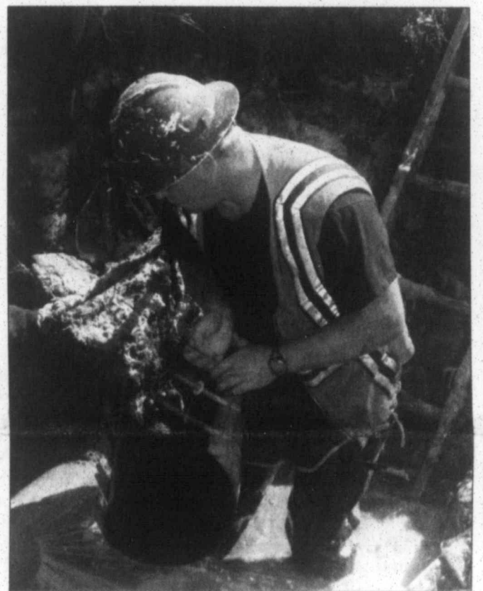
Colby Porter wrestles with a metal sleeve as he prepares to slide it over a broken water main on Coronado Drive.
