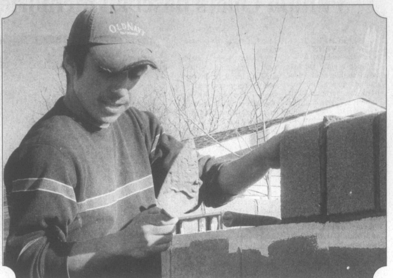
Pampa News photo by MARILYN POWERS Daniel Castillo of West Texas Landscaping wields a trowel to apply mortar to a cinderblock fence he was repairing at a home on 23rd Avenue. The mortar is applied to the surfaces the next block will touch, and the new block is positioned and tapped into place.
