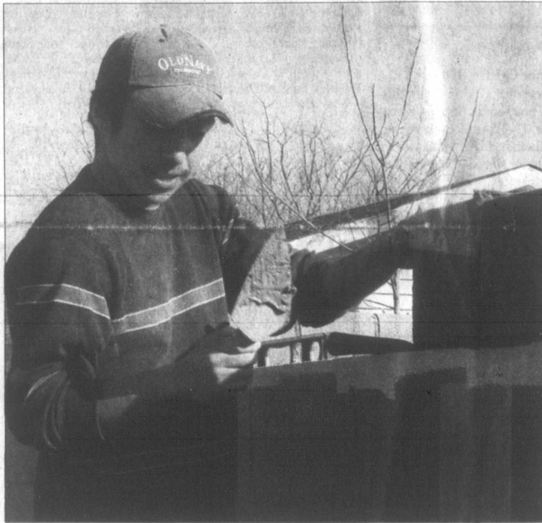
Pampa News photo by MARILYN POWERS Daniel Castillo of West Texas Landscaping wields a trowel to apply mortar to a cinderblock fence he was repairing earlier this week at a home on 23rd Avenue. The mortar is applied to the surfaces the next block will touch, and the new block is positioned and tapped into place.
