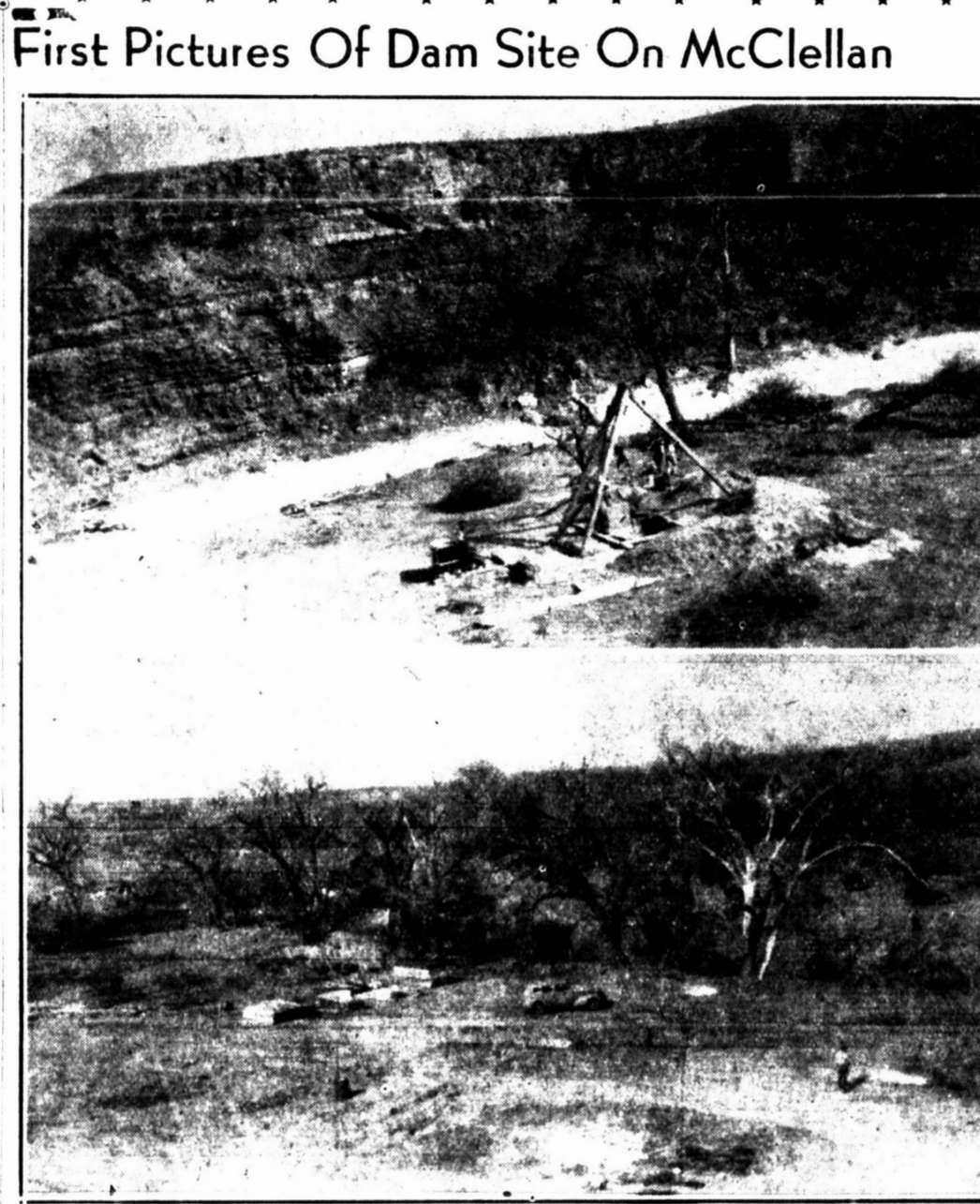
Here are the first pictures of the dam site on McClellan creek. The upper picture was taken from the point of a cliff, not quite as large, but as high, as the one seen in the picture. The dam, about 300 feet wide and 800 feet long, will tie into the bluff seen in the photograph. The dam will extend 55 feet up the cliff. The lake will cover more than 500 acres up the creek which is to the right in the picture. Below the dam is the dam where camps and cabins will be located. A score of men are already working on the dam. In the upper picture may be seen one of the test pits. The approximate cost of the dam will be $300,000.
