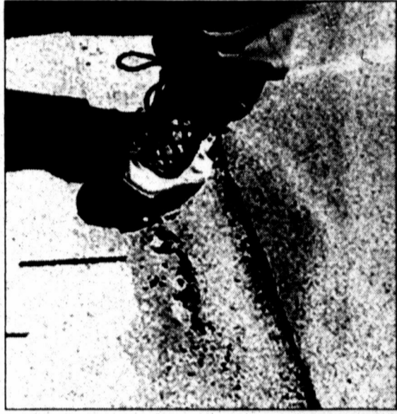
(Pampa News photo by Marilyn Powers) Light pressure with a soft-soled shoe was all it took to expose roof damage on a house in the 2300 block of Rosewood.
