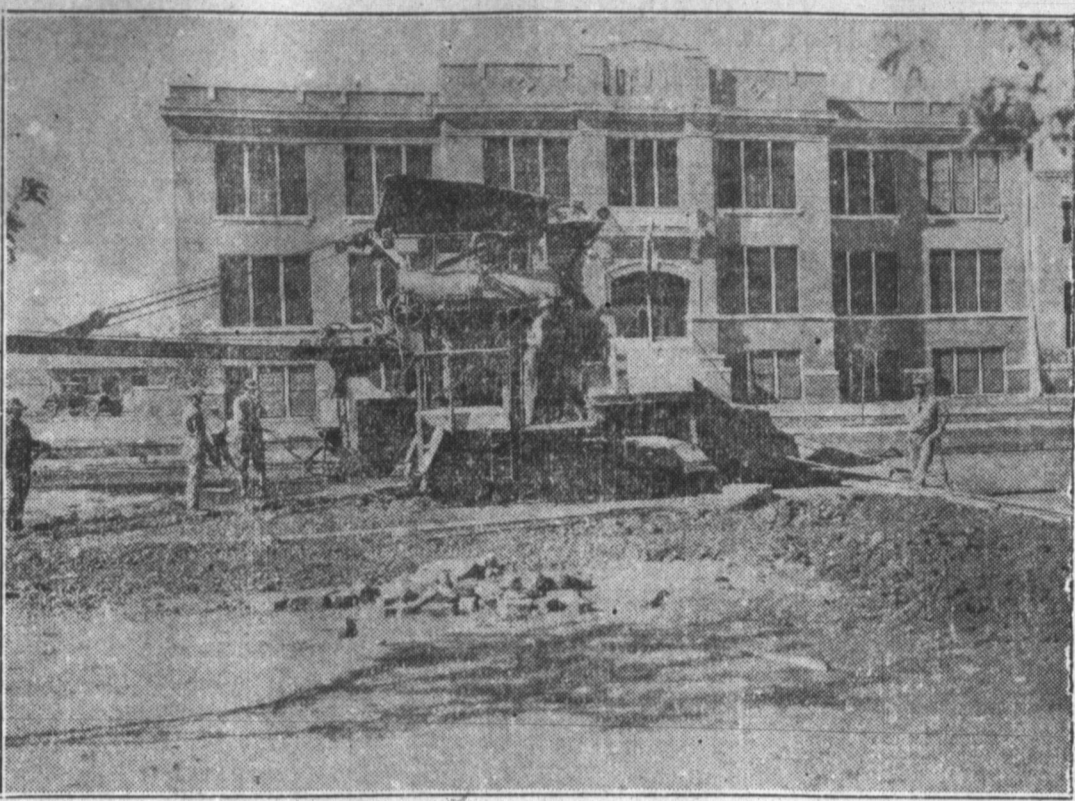
Welcome scenes like the above (in front of Pampa high school) were enacted as Stuckey Construction company poured the concrete for Pampa street paving.
