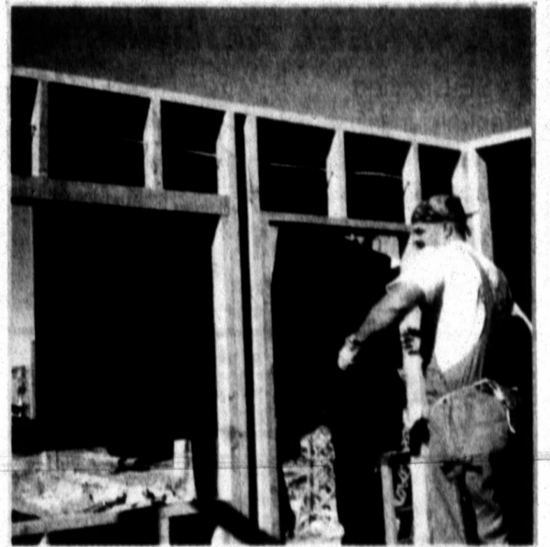
Jeremy Lynan uses his carpenter skills to construct walls for the future home of the family while in Mexico.
