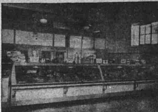
Picture above are two of the modern refrigerated display cases installed as part of the fixtures in the new Safeway store opening here Friday. Top is a 12-foot self-service vegetable display case, made by Koch and refrigerated by the latest type Baker system with thermostat control which assures correct temperature and humidity to retain the natural freshness of perishable items. Customers may obtain their own items through sliding glass panels. Below is a 16-foot refrigerated meat display case—also made by Koch and using the Baker system—which provides the proper temperature and humidity for the preservation of meats. It contains a four-foot compartment for fish and poultry.
