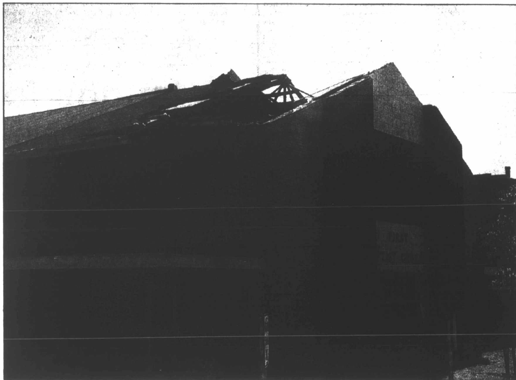
The First Baptist Church of McLean lost a part of the roof in the storm, windows were also broken and an air conditioner ended up on the lawn.
