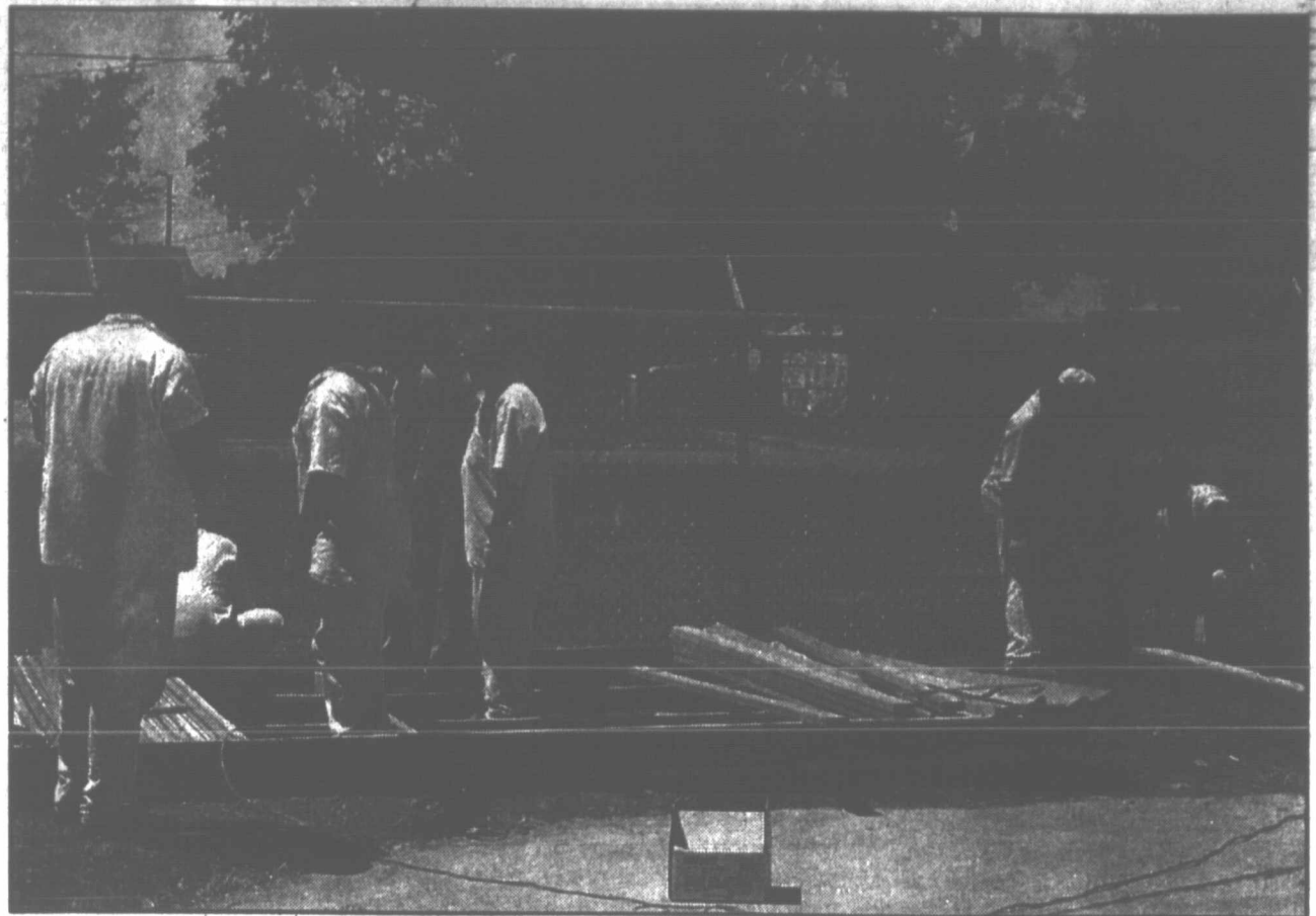
Prisoners from the Rufe Jordan Unit are installing a redwood deck and arbor at the Marcus Sanders swimming pool. In the group are Jarvis Williams, Terry Pickering, Clifford Brown, Rick Nelson of the City Recreation Department, Corrections officer Michael Smith, Robert Martinez, Benjamin Dennis and Terry White.
