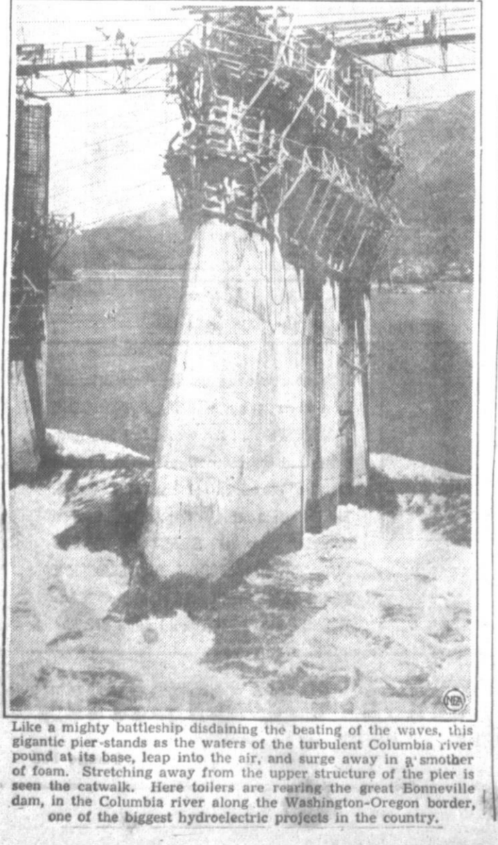
Like a mighty battleship disdainful of the beating of the waves, this gigantic pier-stands as the waters of the turbulent Columbia river pound at its base, leap into the air, and surge away in another of foam. Stretching away from the upper structure of the pier is seen the catwalk. Here toilers are rearing the great Bonneville dam, in the Columbia river along the Washington-Oregon border, one of the biggest hydroelectric projects in the country.
