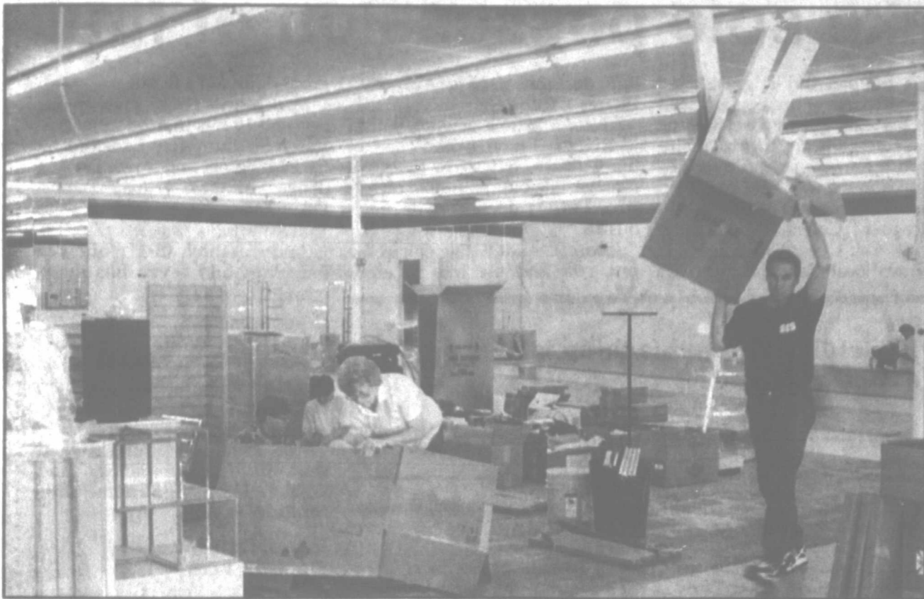
Construction workers are busy getting everything in order at the new Bealls which will open for business on Sept. 25.
