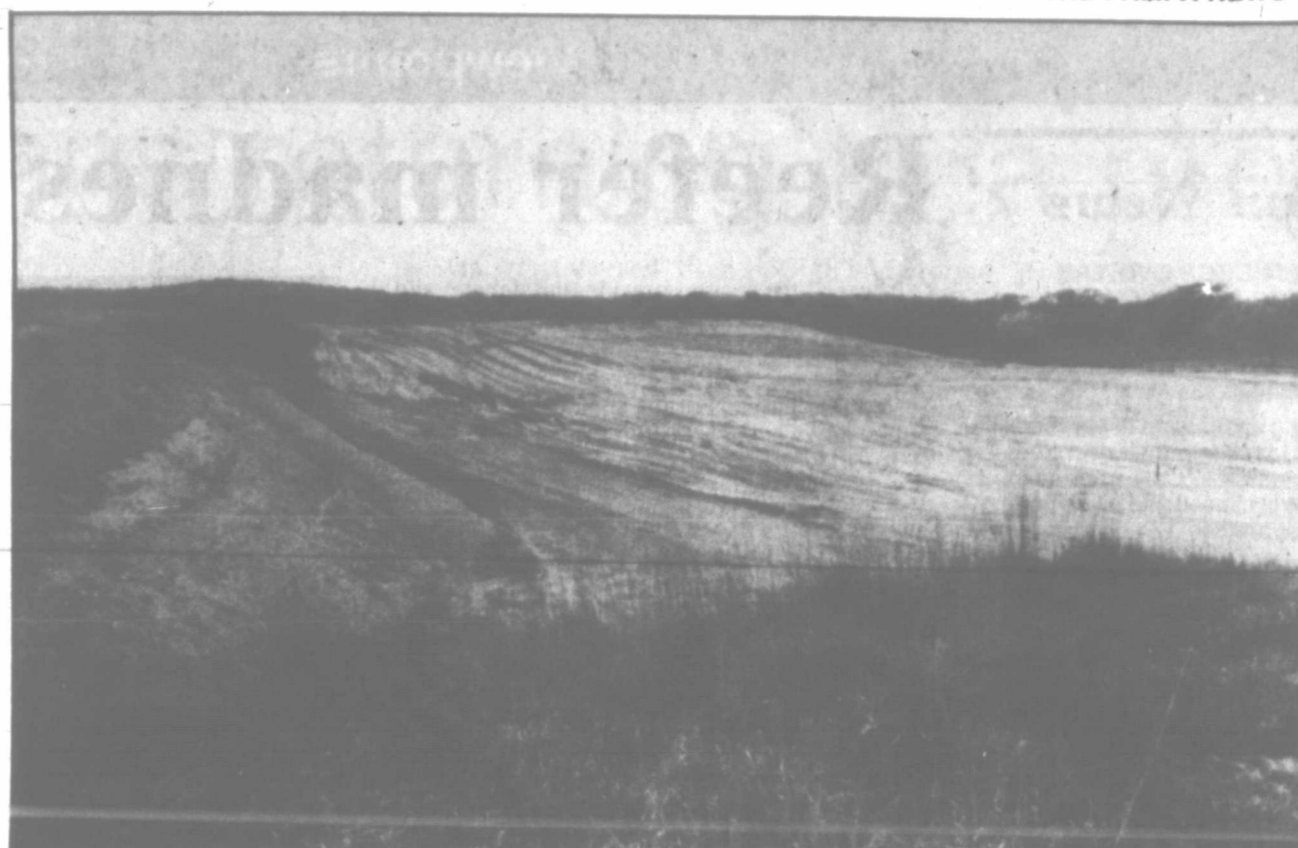
This basin on the northwest side of Lake McClellan is built to hold 160,000 gallons of muddy silt planned for removal from the lake once the lake has mud to remove. On the left of the photo is the retaining wall designed to filter silt so that clear water may return to the ailing lake. (Pampa News photos by Cheryl Berzanskis)
