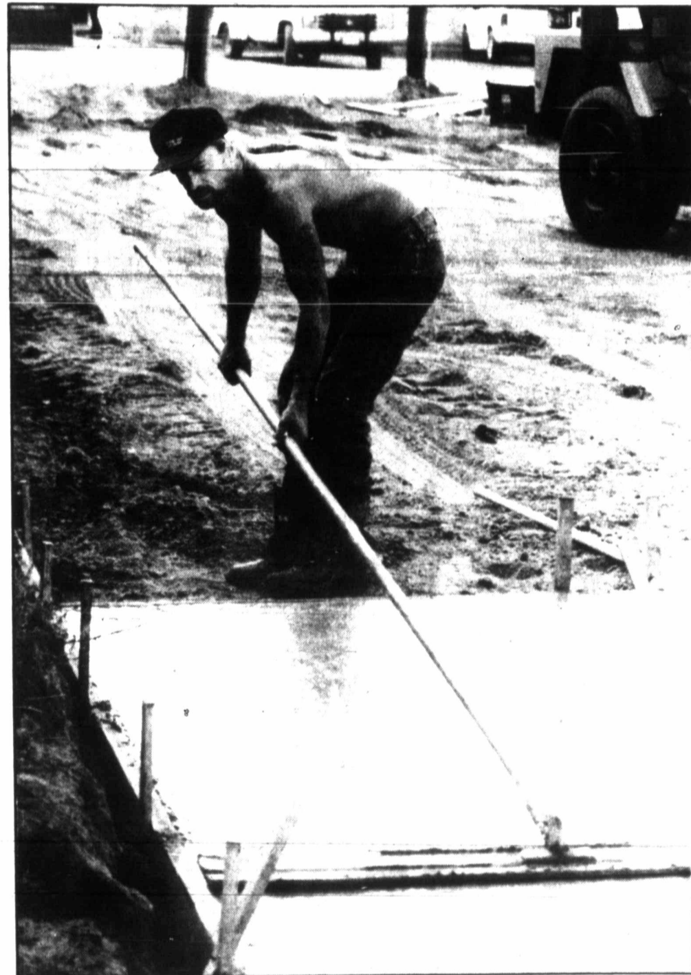
Don Graham pushes a bull float over poured concrete this morning at Auto Zone, 320 N. Hobart, during some construction work at the business. Contractors for the construction are Moore & Moore General Contractors Inc. of La Porte, with some local workers hired for the project. (Pampa News photo by Darlene Holmes)
