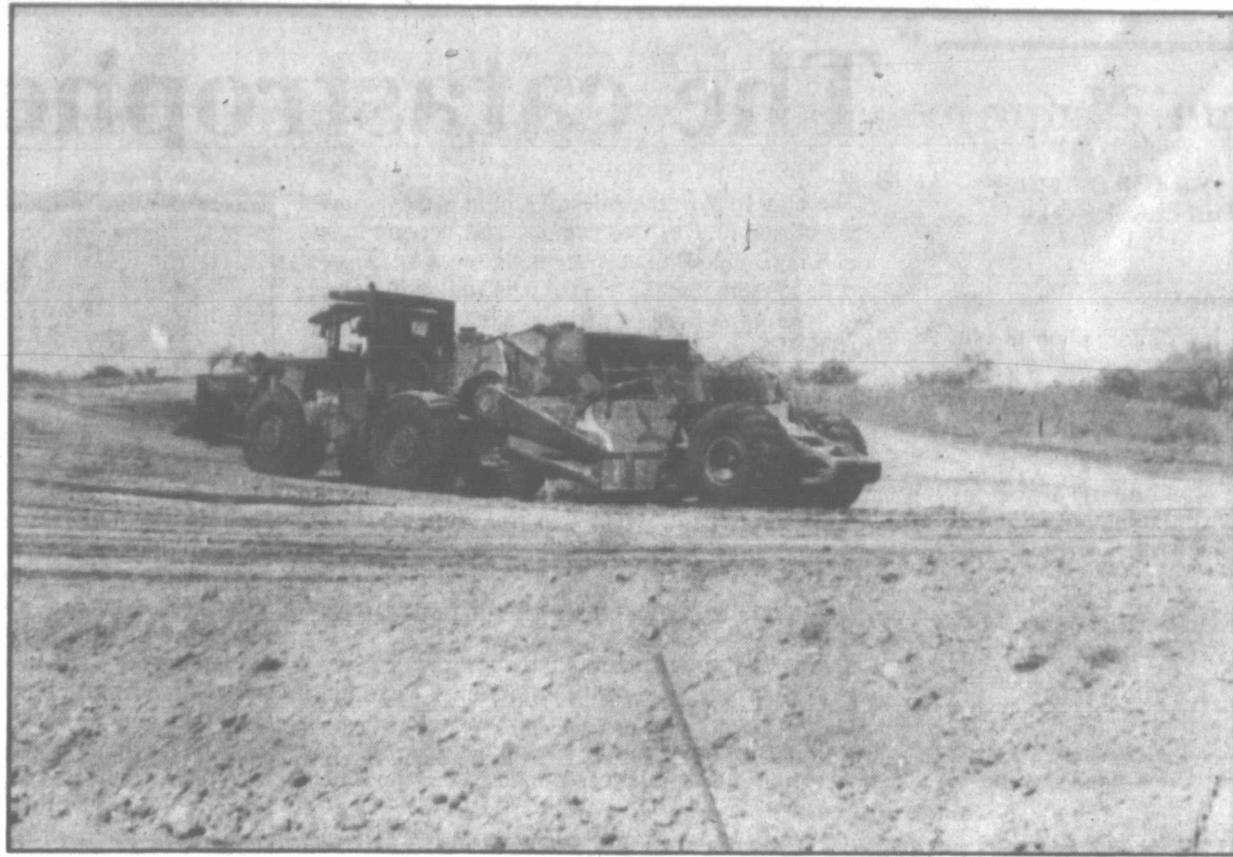
Leland Myers drives a scraper used to compact soil in the silt retaining structure at Lake McClellan. Soil is being layered over a sand and gravel base to create a basin to catch silt from the lake bed. The project involves Gray County employees working to implement a U.S. Forest Service plan to help restore the lake's water area. (Pampa News photo by Cheryl Berzanskis)
