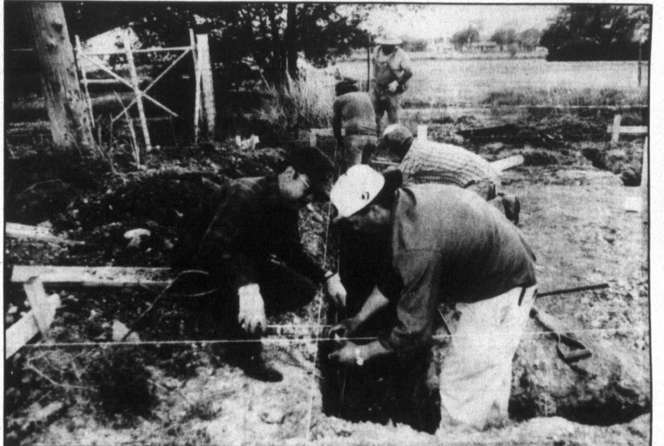
Rick Villarreal (left) and Perfecto Martinez (right) plus other members of Hispanos Unidos pulled together their efforts last night to work on the foundation for a community building that will be set up at 824 S. Cuyler. Once finished, the building, donated by Hoechst Celanese Chemical Group, will serve as a meeting place for Hispanics in the community. It will be a place to teach English as a second language and serve as a place for other activities. Hispanos Unidos plans to build a bigger community building later on. (Pampa News photo by Melinda Martinez)
