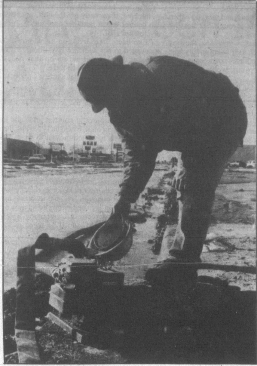
Wes Logan adjusts a water pump along Hobart Street today in an effort to drain water from a construction culvert. Runoff from melting snow delayed the Hobart Street project. (Pampa News photo by Darlene Holmes)
