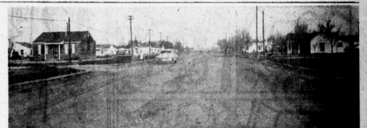
E. FREDERIC —This photo looking east on E. Frederic shows where curb and gutter has been installed, preparatory to the Highway Department's paving the street to a full 60-foot width. In accordance with its standard practice, the Highway Department will pave such highway streets through town from its regular 22-foot width to 60 feet when the property owners along the way install curb and gutter. Curbing will be finished on the few highway streets remaining before the winter is over, and they will be paved in the near future.
