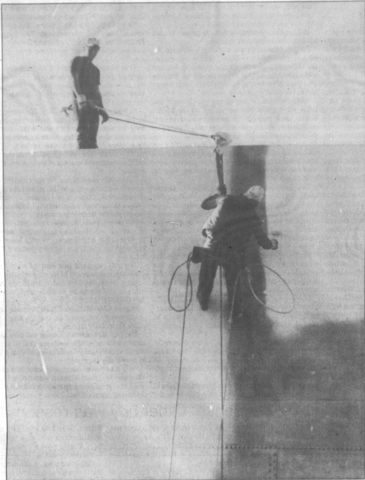
Billy Morgan, top, holds on to a safety rope while Jack Rains braces himself to paint the outside of the city water tank on South Barnes. The two men were busy with the job late last week. They are employees of Corrosion Eliminators of Mineral Wells. (Pampa News photo by Darlene Holmes)
