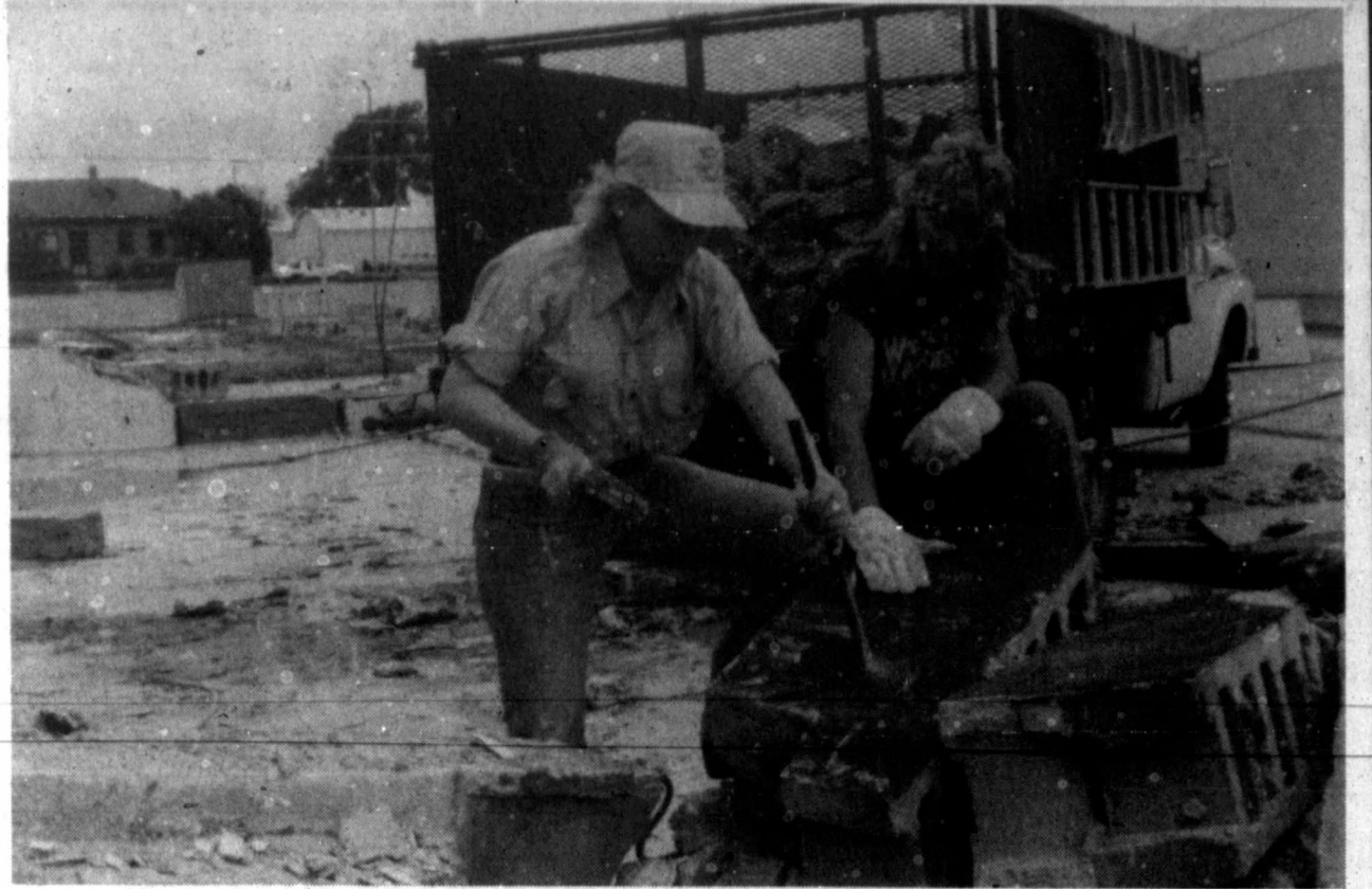
Cathy Teague, left, and Connie Skinner clean and haul off blocks from a building at 512 S. Cuyler St. that was torn down for the First Assembly of God Church. The church plans to use that land as a parking lot that will be adjacent to the church. (Staff Photo by Darlene Holmes)
