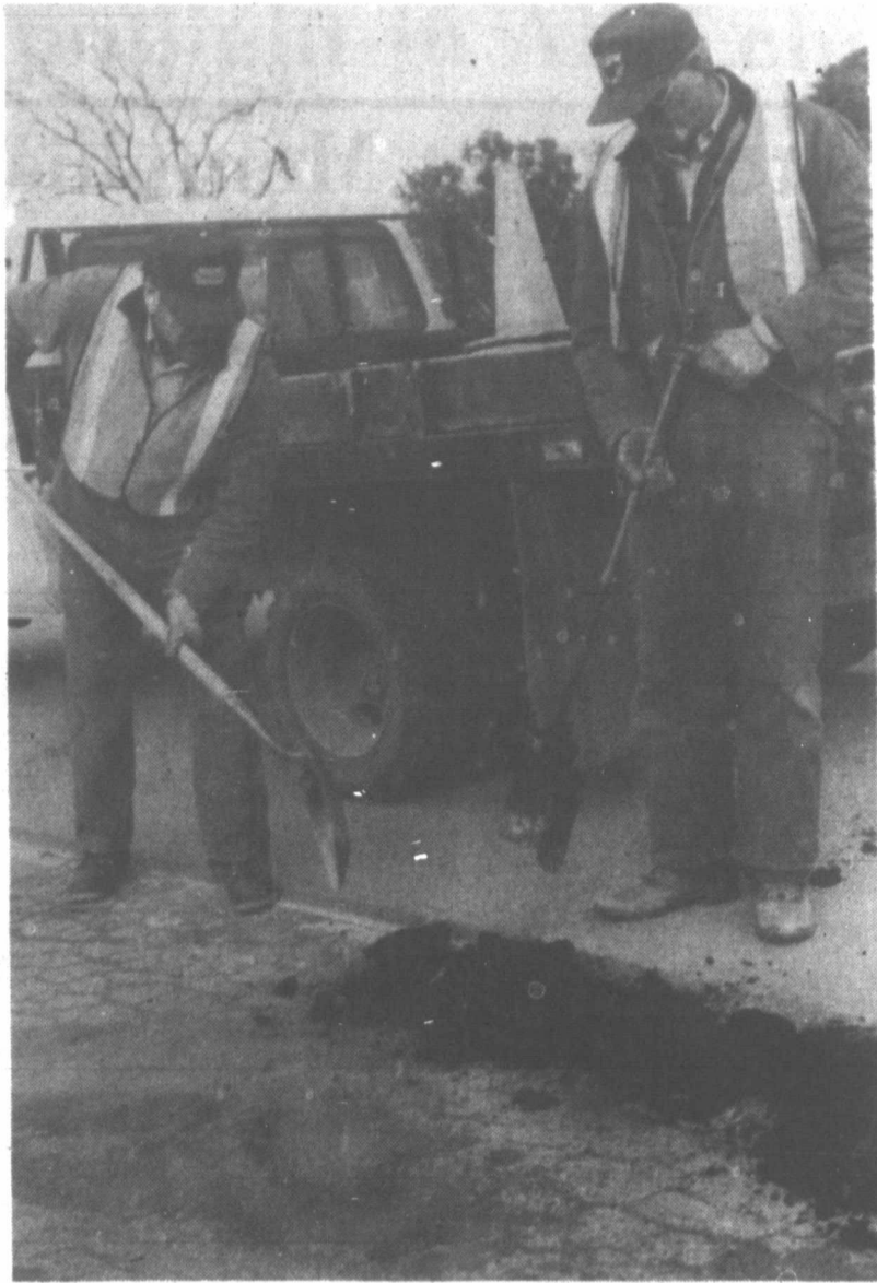
(Staff photo by Cheryl Berzanskis) City of Pampa employees John Oxley, right, applies heat as Eddie Guerra shovels asphalt in the 2400 block of Duncan Friday as they fill potholes.
