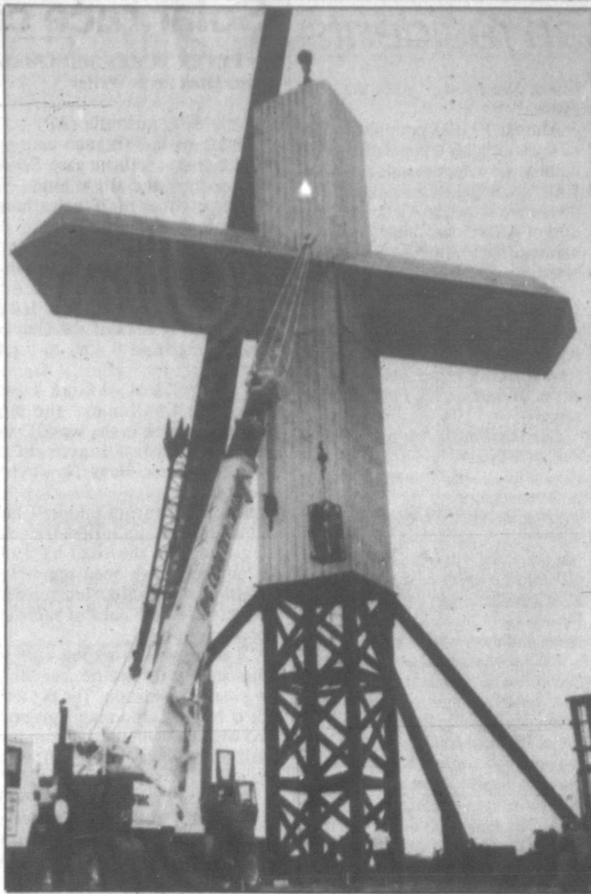
Construction workers install panels on a 10-story cross being erected near Ballinger on Oct. 8. The cross, funded by James Studer, is built as a tribute to God.
