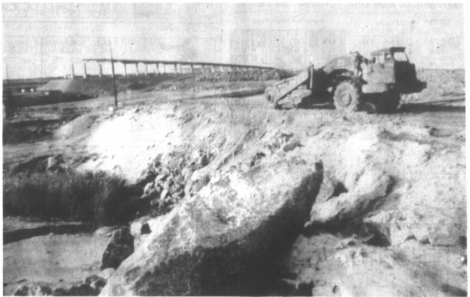
A highway bridge (background) will span one of the two locks for ocean going ships on a dam across the Gulf of Finland near St. Petersburg, Russia. The dam has trapped polluted water and sediments laden with heavy metals. (National Geographic photo)
