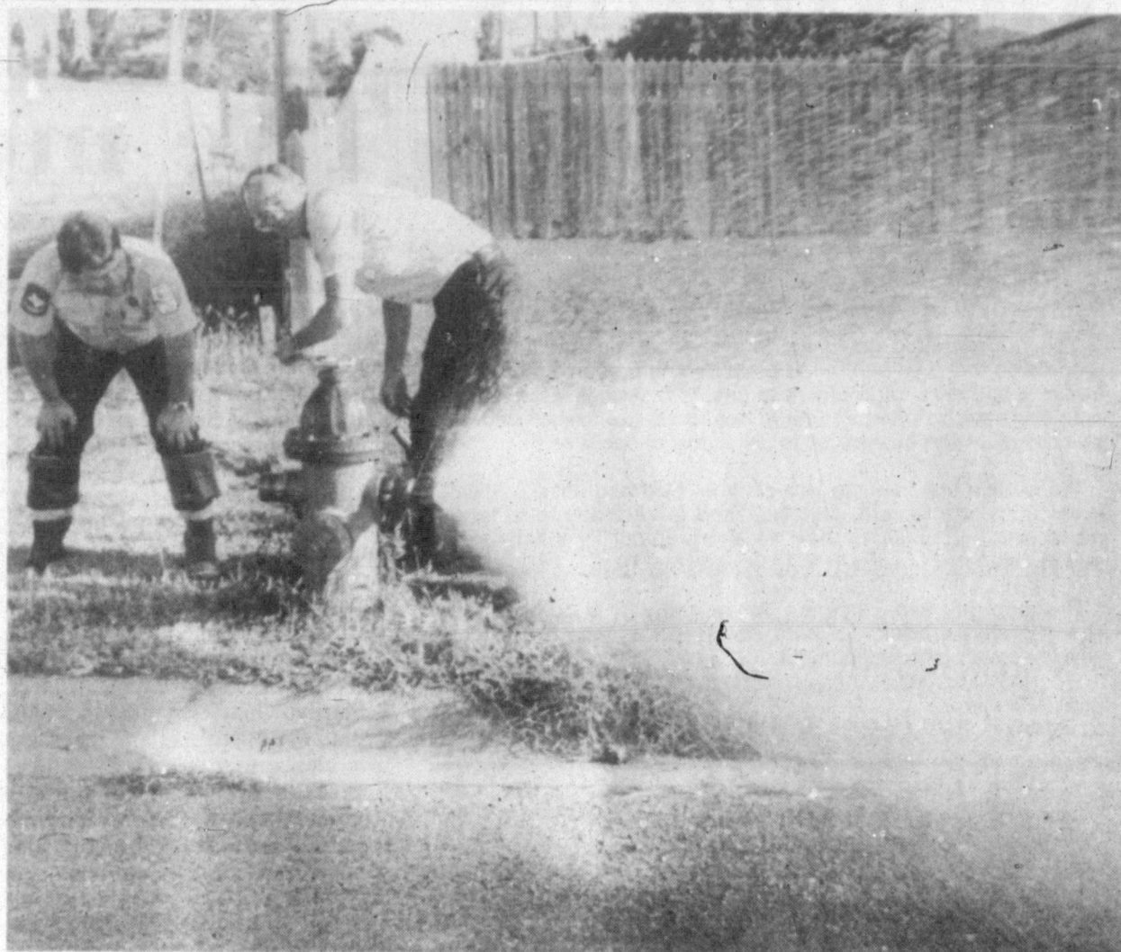
Firefighter Gary Parks, left, and Driver W.D. Thomas flush and check the water pressure on fire hydrants on the east end of 23rd Street. The fire department annually checks fire hydrants. (Staff photo by Daniel Wiegner)
