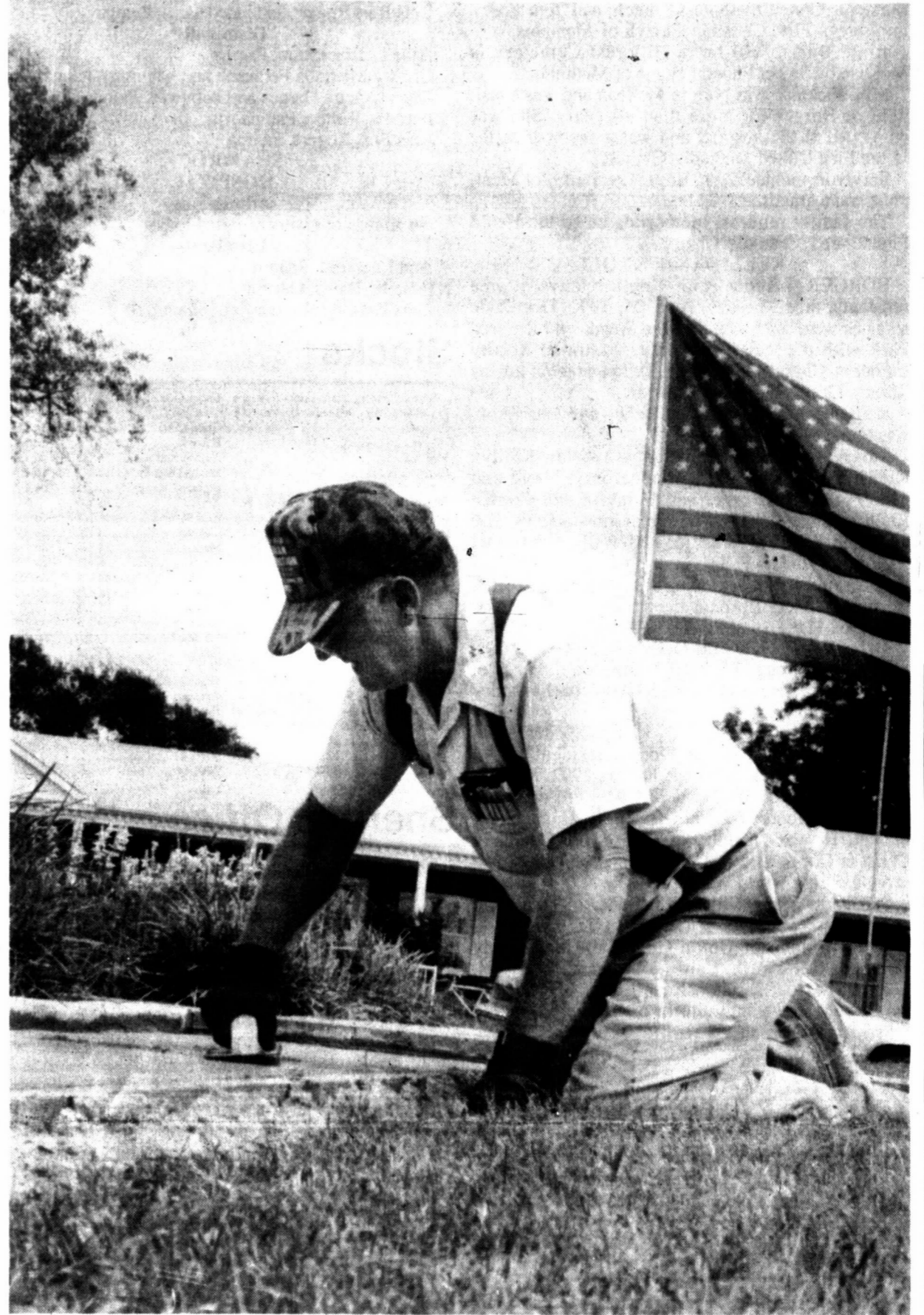
Bill Hagerman smooths cement for additional brick space at Memorial Park on Hobart street Wednesday. The new space will hold over 300 names of veterans who have served in the U.S. military.
