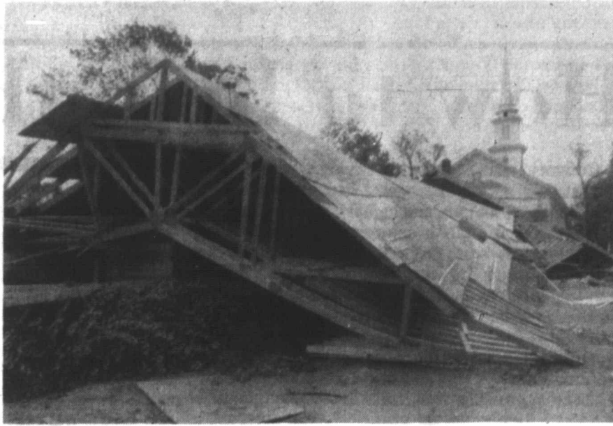
An addition to the First Congregational Church in Falmouth, Mass., collapsed under the winds of Hurricane Bob as it hit Cape Cod on Monday.
