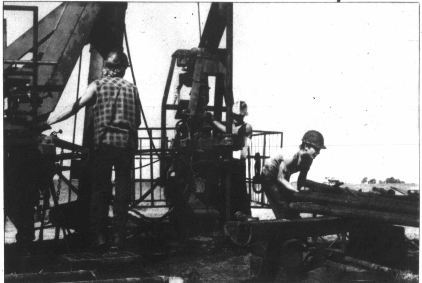
These employees of Curtis Well Service are running tubing and working on a pulling unit at an oil well west of Pampa.
