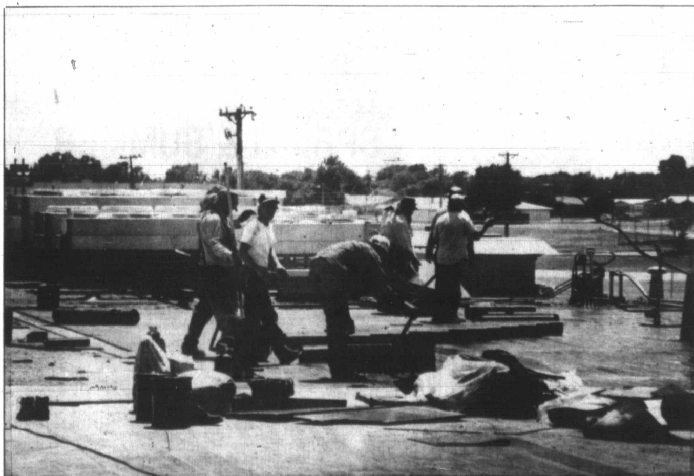
Hot tar roofing is probably the quintessential example of "hot work". These men are working with molten tar on a sun-baked roof at Pampa Mall. Job foreman, Buzz Lockridge, said that despite the searing heat, he prefers his work to indoor jobs. The men drink a lot of Gatorade and ice water. They all wear sunglasses. He said that he can tell when the men are getting too hot because they begin to slow down.
